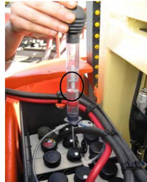
Figure 8-4. Measuring Electrolyte Specific Gravity
